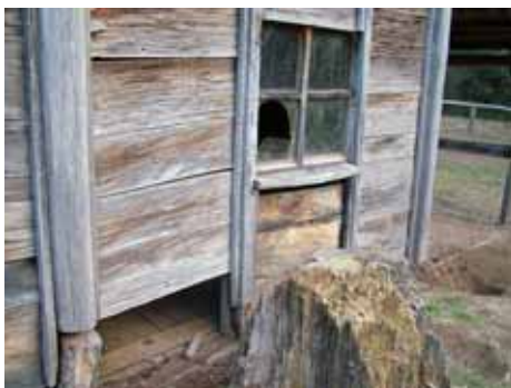
The missing slab and broken window, photo by Fleur Smith ParksVic.
